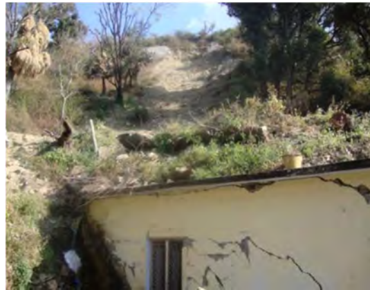
A view of the damaged house due to the slide in East direction.
